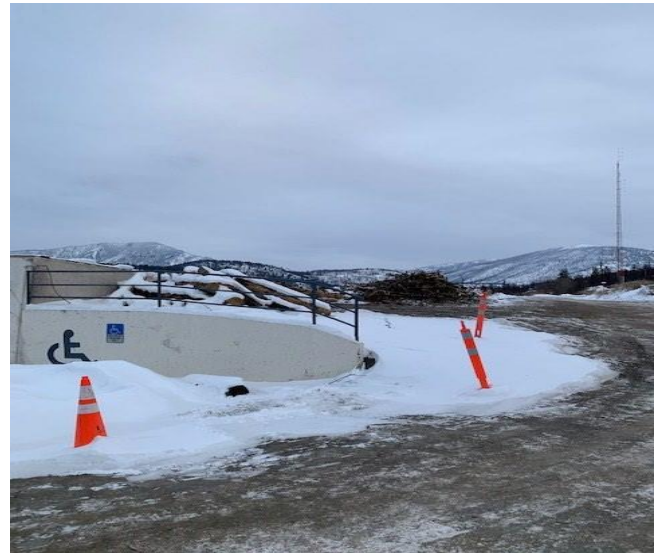
Photo 2 – Metal Debris 90% removed, some retaining walls remain pending geotechnical evaluation
