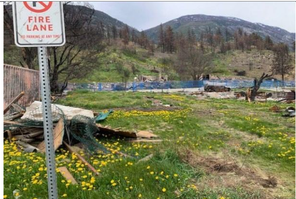
Figure 8 – Zone 2 Lot 144 debris removed
